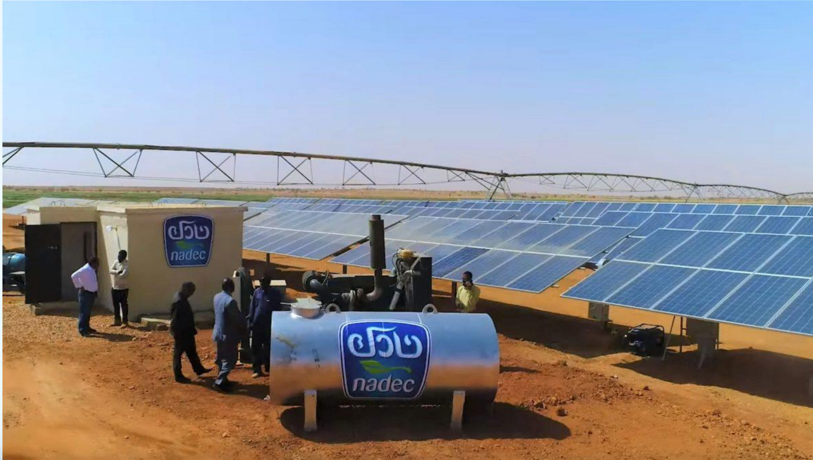
Nadec Project -30MW Location :Saudi Arabia
