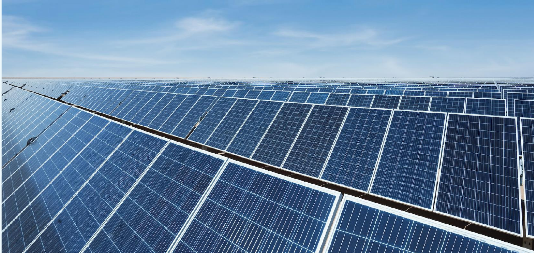
Laila Project Location :Saudi Arabia. Project : Ground-Mount 13 MWp
